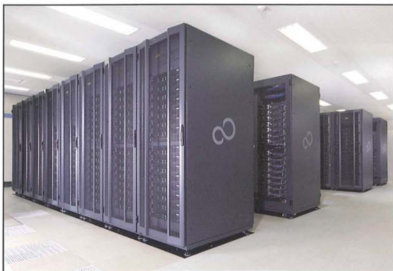
Fujitsu PRIMERGY RX300S7
